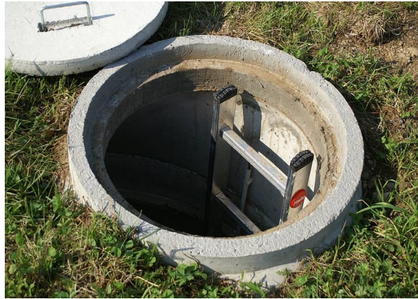
Figure.26 Ground water recharge well at public recreation center
