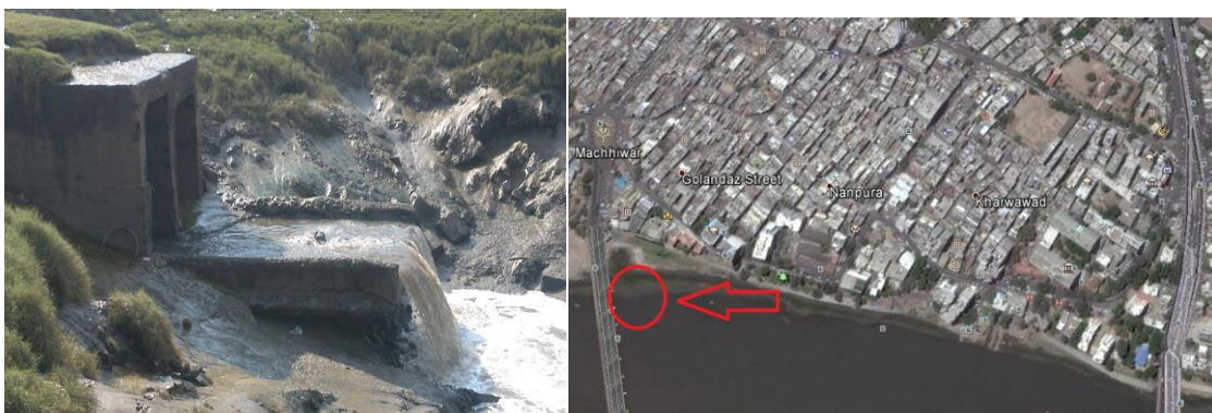
Figure.7 L7 flood gate, D/S of Makkai Bridge
