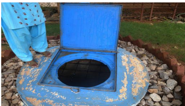
Figure.25 Ground water recharge well for domestic use
