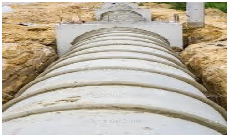
Figure.27 storm water storage line
