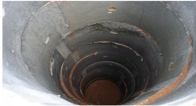
Figure.18 Ground water recharge well
